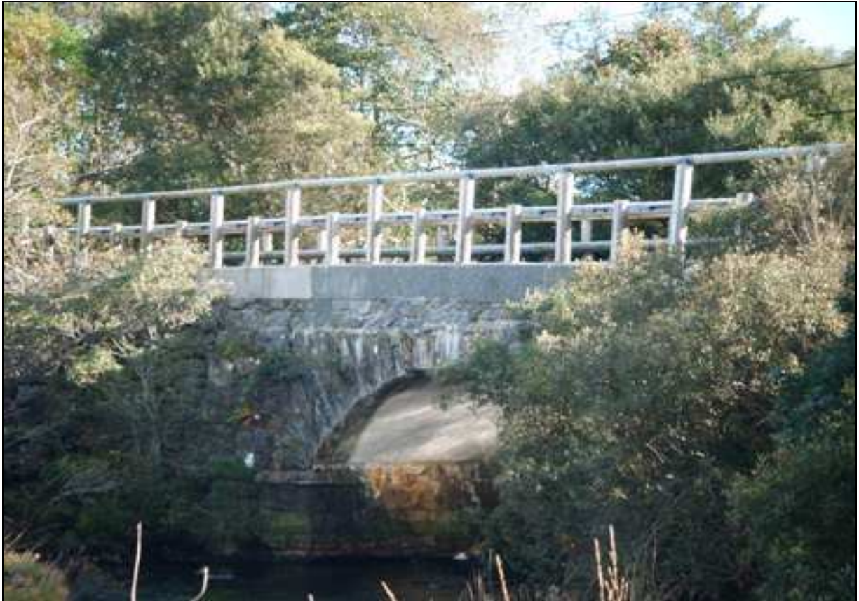
Plate 15: Bridge GC-N59-029-00 over the Owentooy River east of Recess village at Chainage 244900
